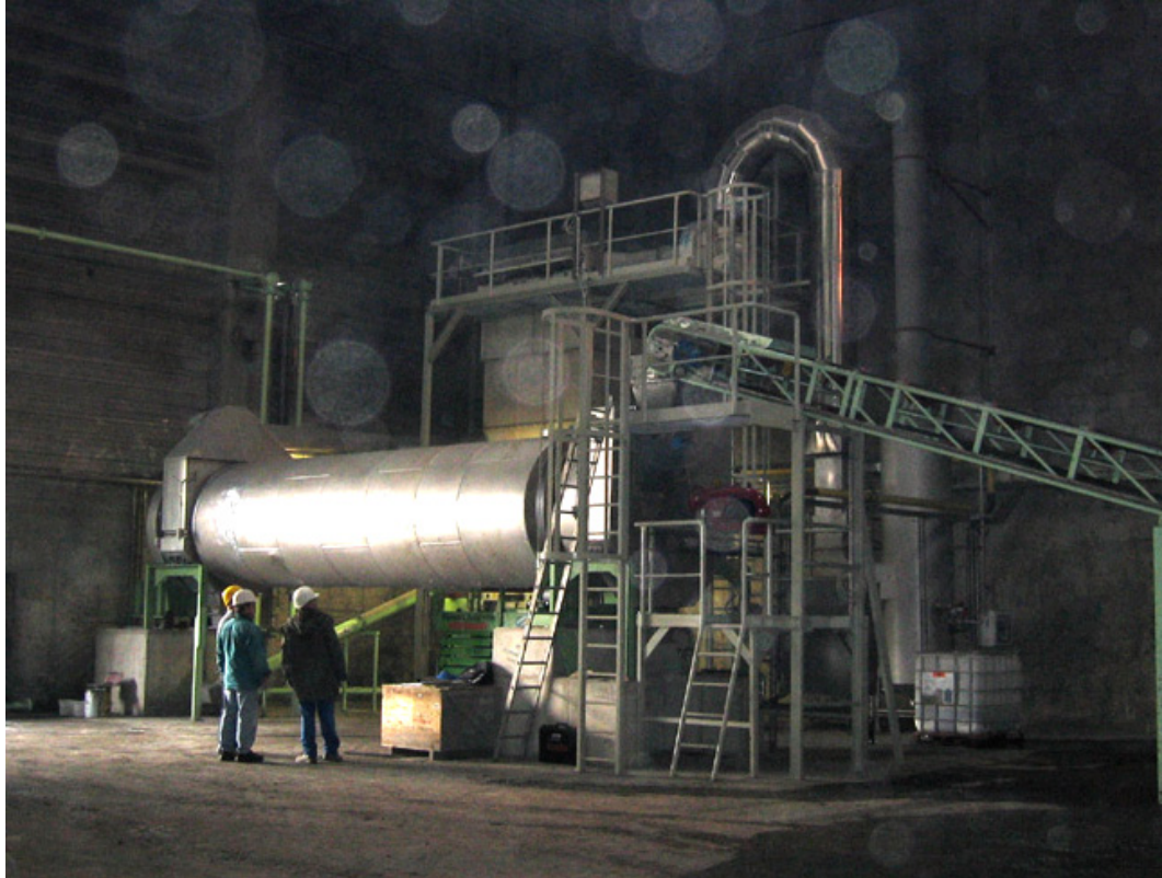
Picture 4: view of the SEROX drying facility of ALSA Hannover
